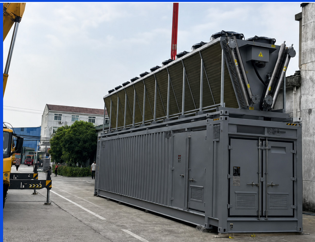
Containarised Direct Immersion Cooling
